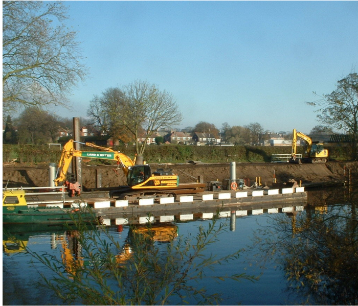
River bank repairs at Clifton – piles being set into river bank, and accumulations of silt being stripped off bank tops
